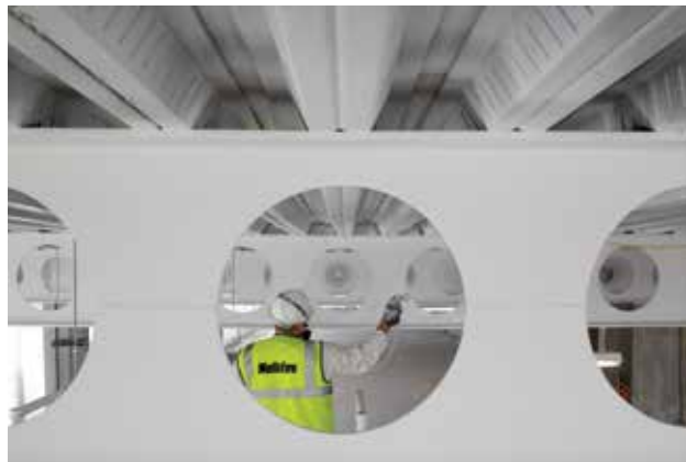
E. FIRE PROTECTION
